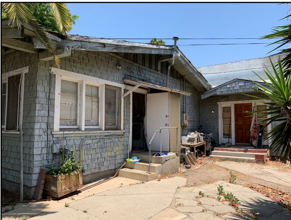
Figure 3.1.3. Overview of southeast (rear) façade of 1642 South Central Avenue, view facing north (SWCA, June 2021).
