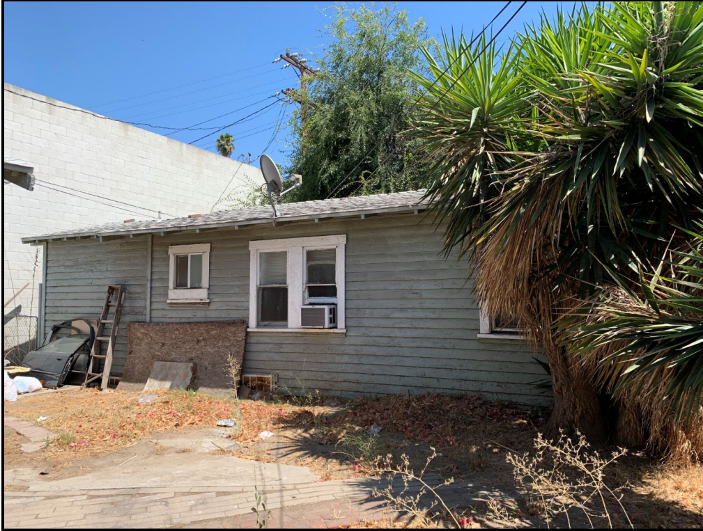
Figure 3.1.6. Northwest façade of 1608 Gardena with the 1953 addition at the north end, view facing east (SWCA, August 2021).
