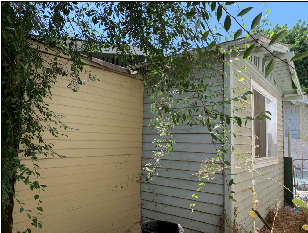
Figure 3.1.5. Northeast (rear) façade of 1608 Gardena with the 1953 addition, view facing west (SWCA, August 2021).
