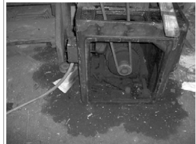
5. View of de minimis oil staining under an abandoned lathe in Building 1.
