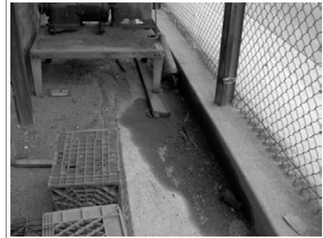
6. View of de minimis oil staining under an air compressor located south of Building 1.
