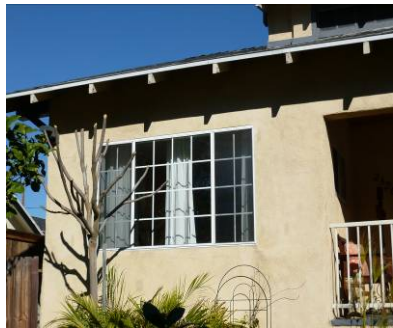
Not this: mullions were removed and flush window was installed instead of recessed
