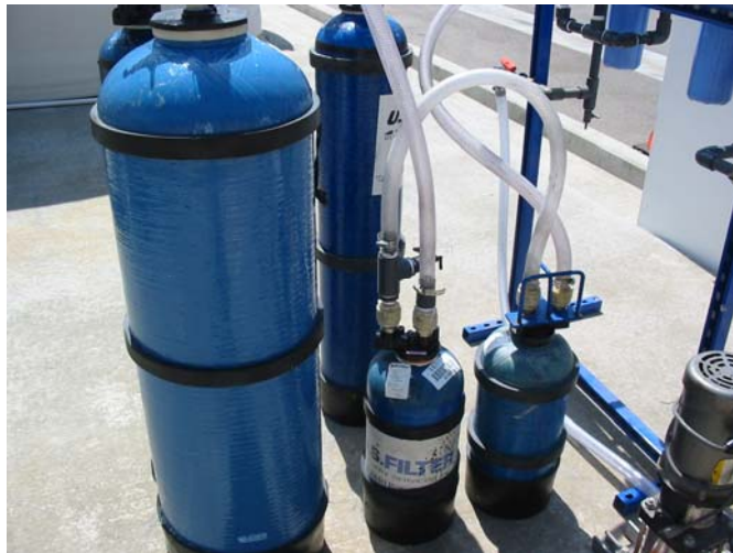
USF/R&H WBA System (cation exchange column for pH control on left, followed by two small lead-lag WBA resin canisters in the foreground)
