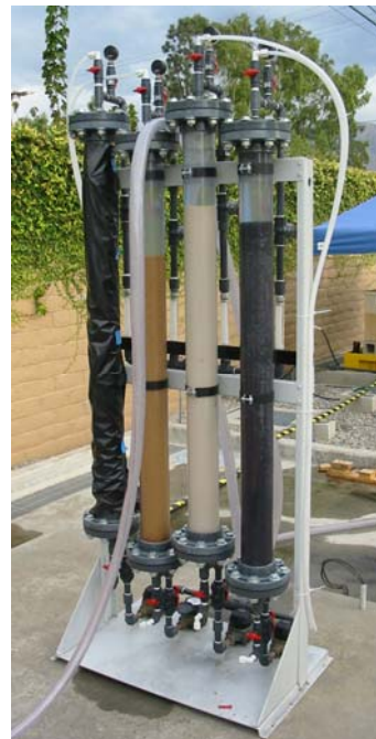
Calgon Pilot Unit (Trial 2 shown; GAC in right-hand column)
