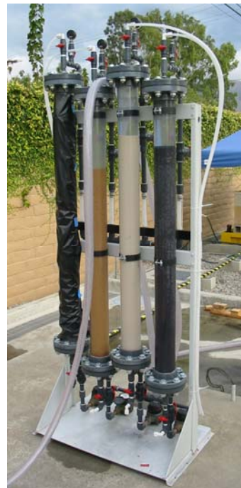
Calgon Pilot Unit (Trial 2 shown; SBA resin in middle two columns)
