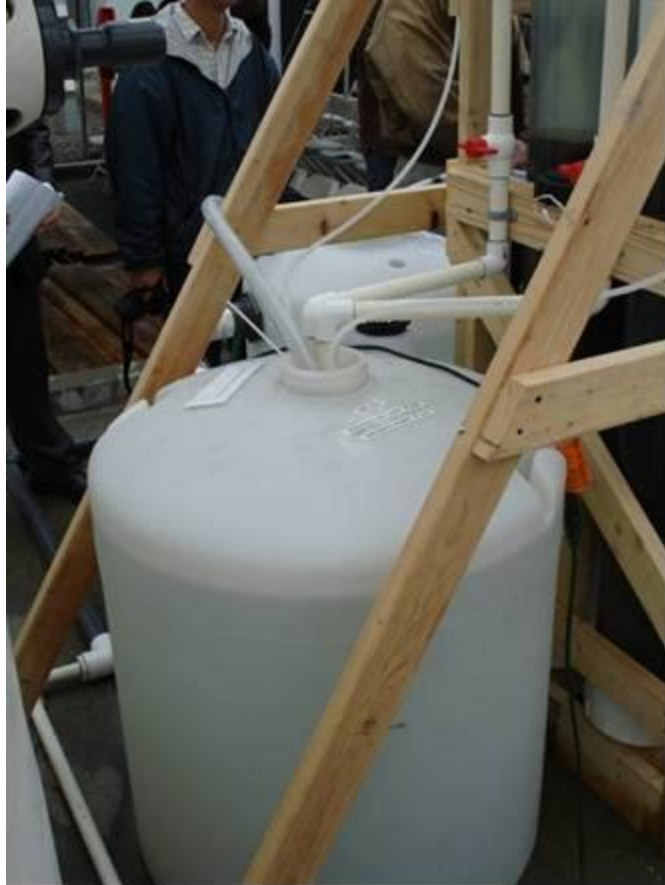
Figure B-10. Backwash Water Holding Tank
