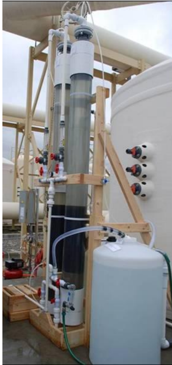
Figure B-6. Parallel Filtration Columns and Effluent Tank
