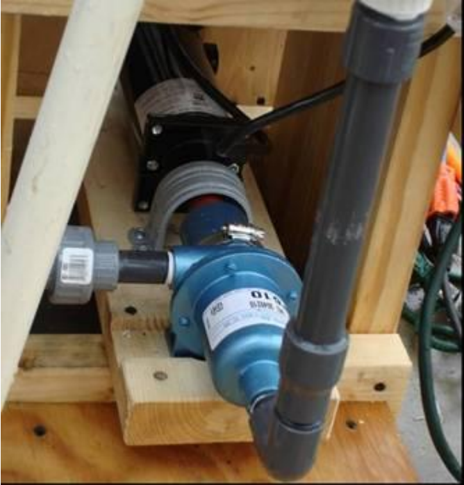
Figure B-5. Progressive Cavity Pump Between the Rapid Mix and Filter Columns
