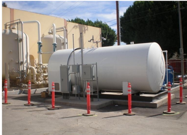
PHOTO 1 - CARBON DIOXIDE SYSTEM WITH ION EXCHANGE VESSELS
