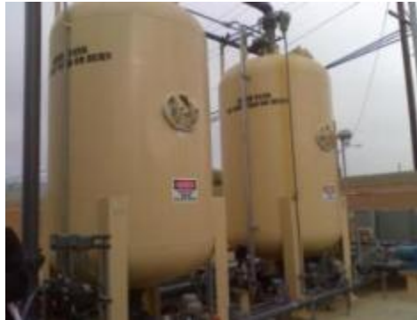
PHOTO 4 - VERTICAL PRESSURE VESSELS
