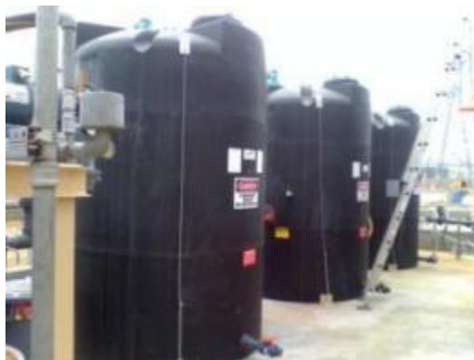
PHOTO 3 - REDUCTION TANKS WITH MIXERS
