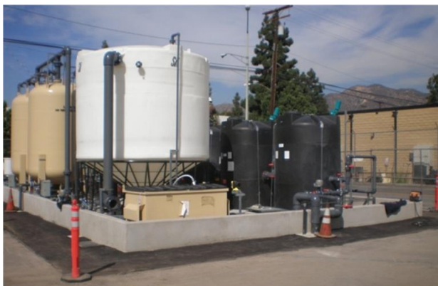
PHOTO 2 - RCF DEMONSTRATION-SCALE SYSTEM
