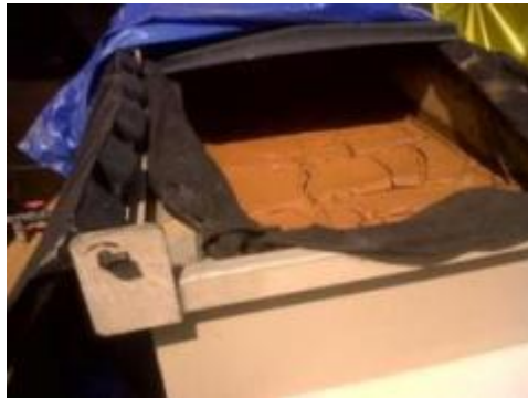
PHOTO 5 - PASSIVE SLUDGE DEWATERING SYSTEM - SLUDGEMATE
