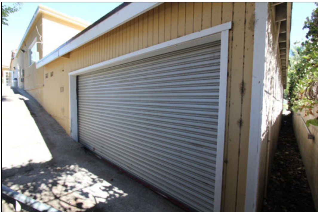
Fig. 31: 3067 E. Chevy Chase Drive, north elevation, garage north entrance, view southeast (Chattel, 2014)
