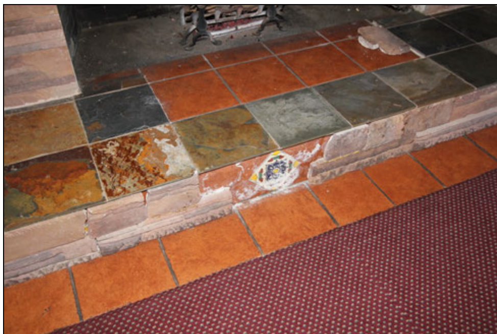
Fig. 53: 3067 E. Chevy Chase Drive, first floor, east banquet room fireplace footing detail (Chattel, 2014)
