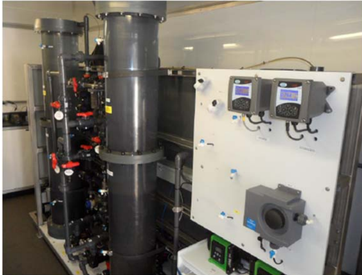
Figure 5.2 Photograph of Cleanit® pilot unit
