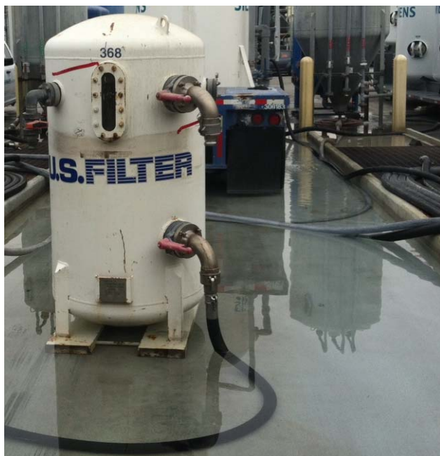
Figure A.1 Resin preconditioning vessel
