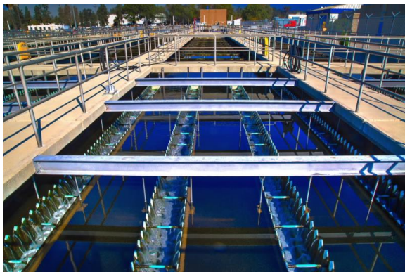
Figure 2.13: Wastewater Treatment at LAGWRP
