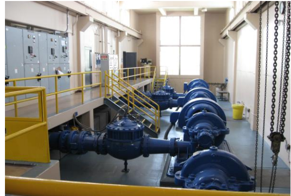
Figure 2.11: Grandview Pumping Plant
