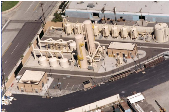
Figure 2.10: Glendale Water Treatment Plant
