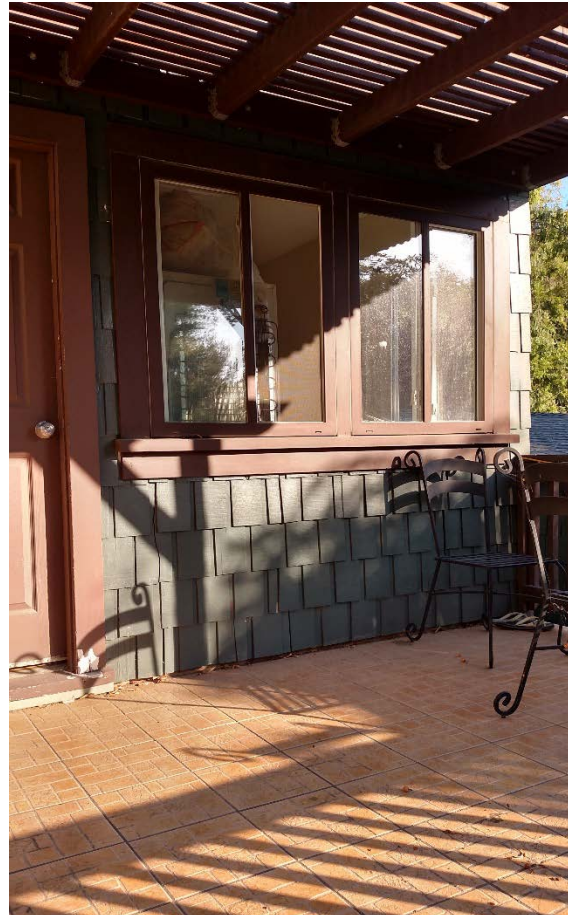
PHOTO 2. Close-up view of the front porch of the back house showing wood shingle siding and wood framed windows. The porch is covered in a lattice-like open wooden structure.
