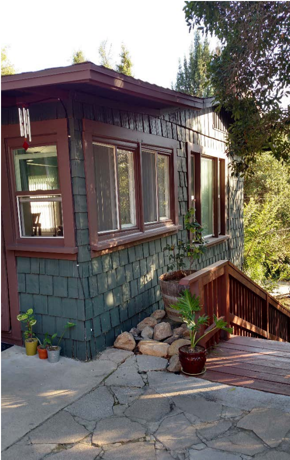
PHOTO 1. View of front home showing the wood shingle siding and the wood frame windows. The minimally pitched roof has a short overhang. Windows are double hung or fixed. Some windows have newer vinyl inserts. Only about 10 percent of the windows are fully original.
