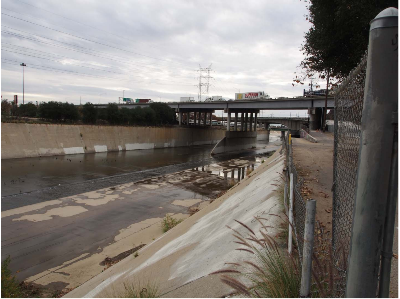
Photo 20: Depicts the transition at the southern end of Segment 5 to concrete bottom of Segment 6, where the River forma a thin sheet of water at the edges of a deeper, fast moving center channel. Photo was taken from the bike path facing southeast.
