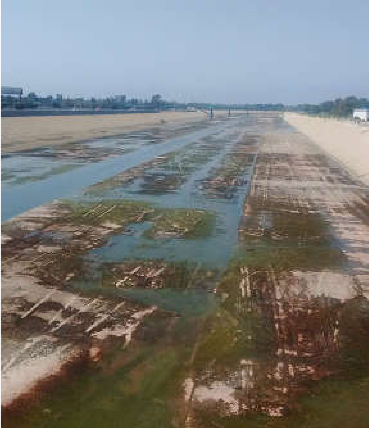
Figure 3. Algal mats fed by overflow from the low flow channel (Segment B)
