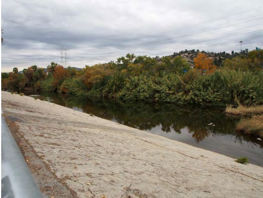
Photo 18: Depicts the BWT in the southern-central portion of Segment 5. Photo was taken from the bike path facing northeast.
