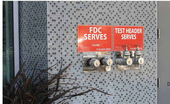
ABOVE: Utilities such as standpipes, fire department connections, and utility boxes are essential to building operations. Utilities shall be incorporated into the building design to the greatest extent feasible, including wall mounted devices, to avoid freestanding obstructions in or near the right-of-way, or visual clutter within landscaped areas or setbacks.
