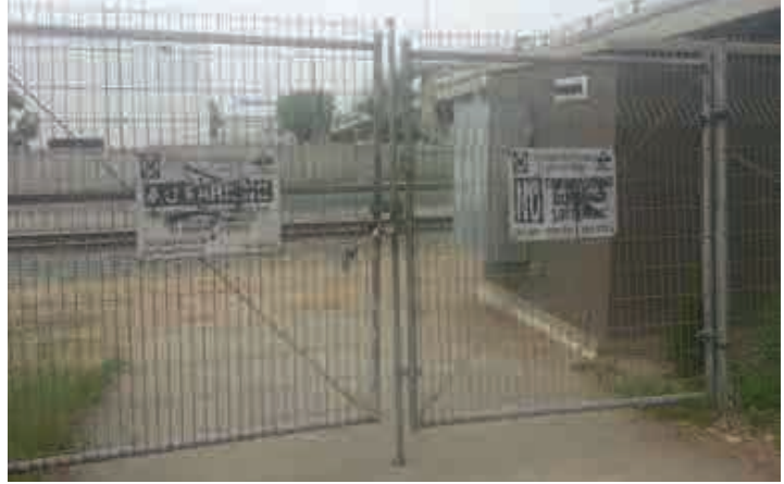
1.7 Unclear Safety Signage
