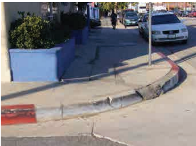
3.7 Lack of curb cuts
