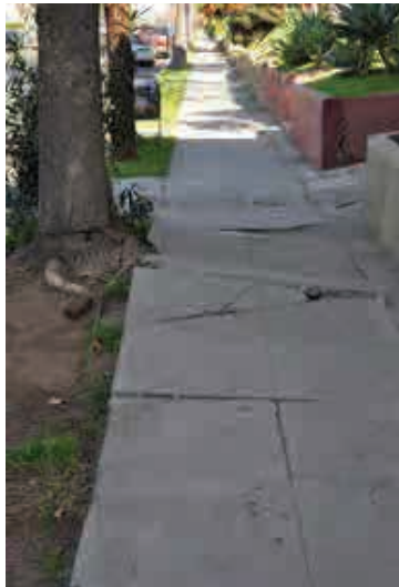
3.1 Buckling sidewalks / inadequate sidewalk width
