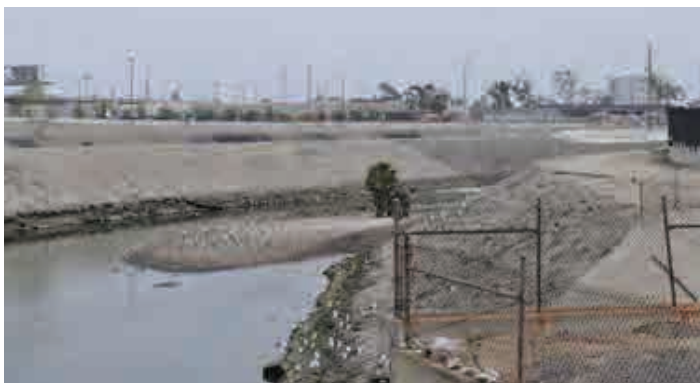
2.5 Problematic drainage infrastructure bordering station
