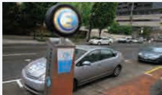
Curbside electric Vehicle charging station, Portland, OR
