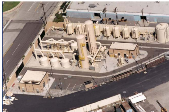
Figure 6.5: Glendale Water Treatment Plant
