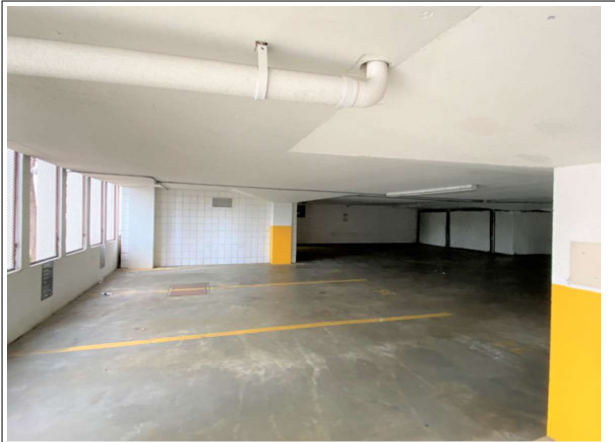
Figure 2: Parking Garage interior view north. Note the fitted screens in the exterior openings (left) archaic stack bond endwalls (center and right), and square, full height support columns at center and right with yellow bases. Photograph January 2022.
