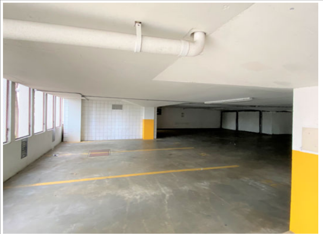
Figure 2: Parking Garage interior view north. Note the fitted screens in the exterior openings (left) archaic stack bond endwalls (center and right), and square, full height support columns at center and right with yellow bases. Photograph January 2022.
