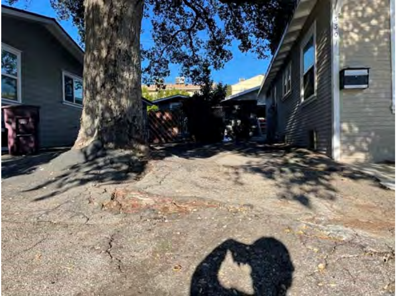
Figure 2: Tree 1 has caused significant uplift and displacement to the existing asphalt driveway. There is limited space between the tree and the house, so the driveway must be retained in place to permit vehicular access. There is very little space for tree protection fencing.
