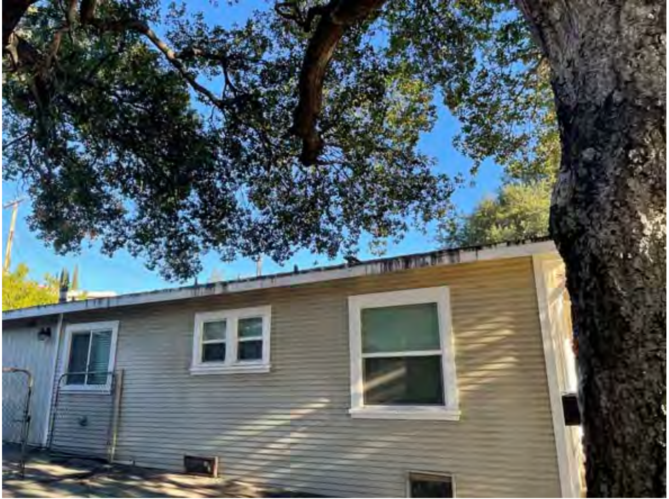
Figure 6: The canopy of Tree 1 is growing within 5 vertical feet of the roof of the adjacent house. It will be pruned for clearance over the roof.
