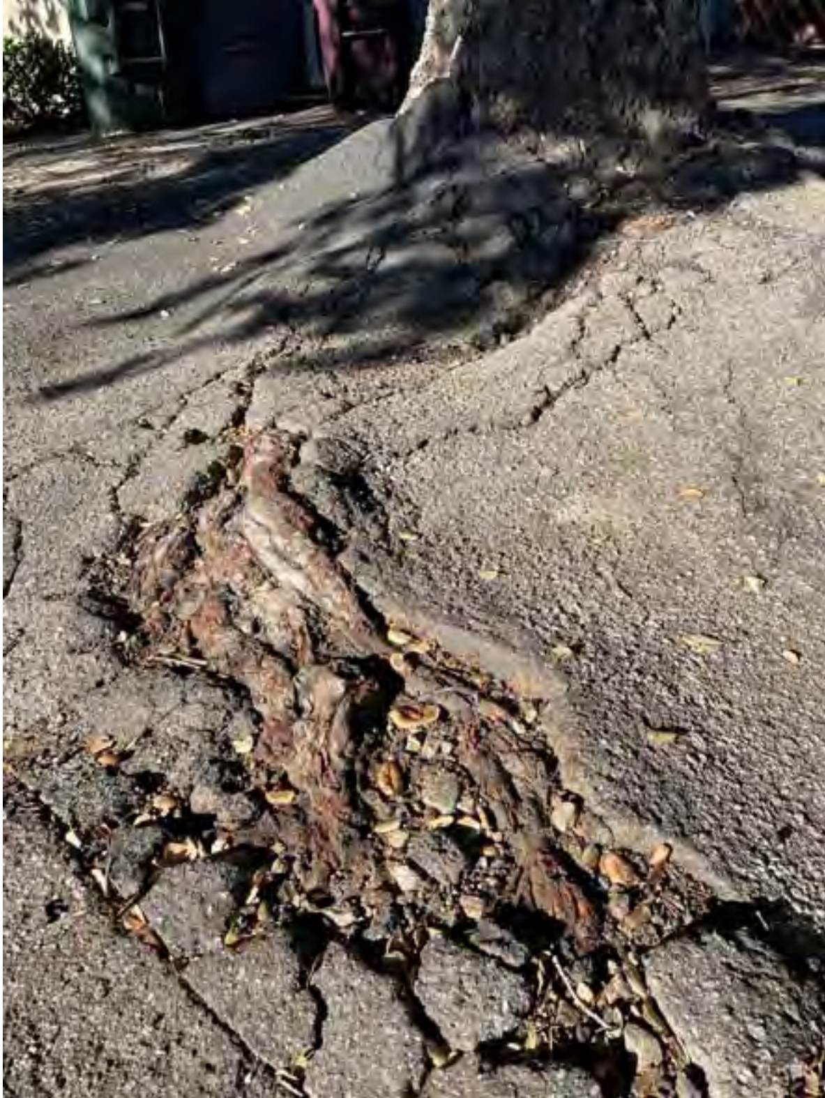
Figure 5: One of the roots of Tree 1 that had breached the upper surface of the asphalt driveway. This root had sustained mechanical injuries from vehicles driving over it.
