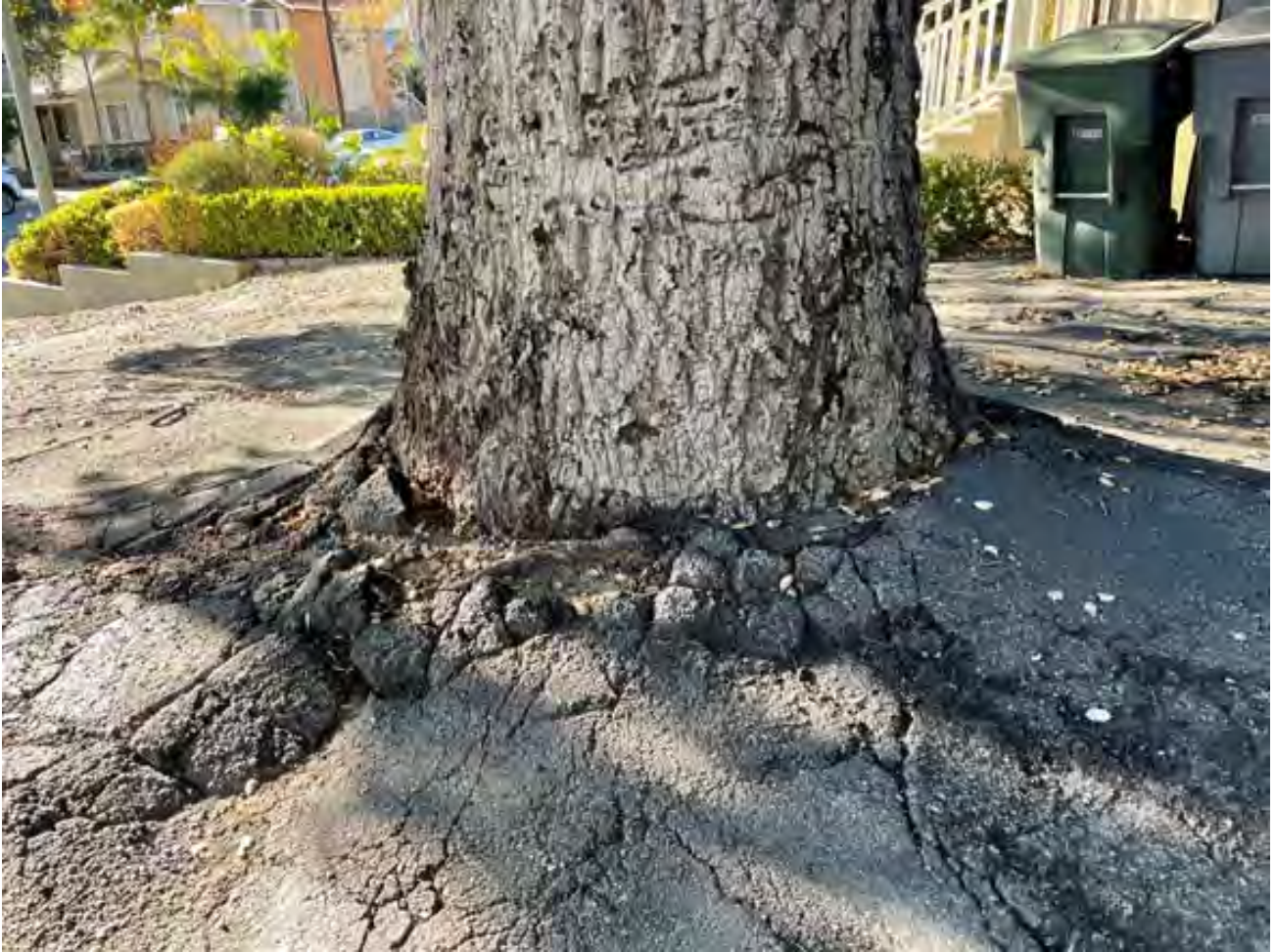
Figure 3: The entire root crown of Tree 1 was paved with asphalt. The driveway is so narrow that the asphalt must be retained in place to permit use of the driveway, despite the suboptimal condition for the tree.
