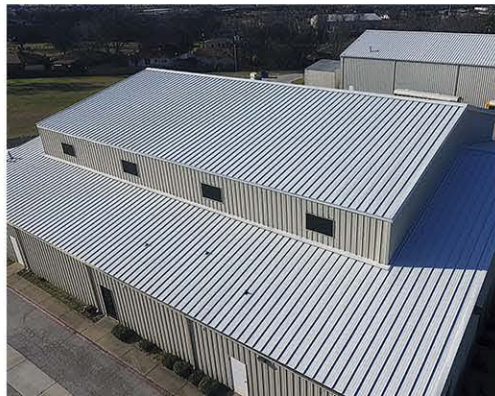
⑪ Standing seam metal roof (Metal Sales, Clip-Loc Metallic Silver)
