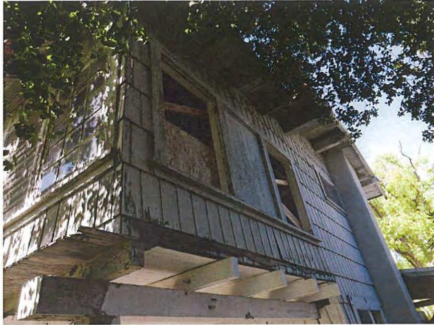
Figure 3. Detail of Rear Second Floor Addition, 534 N. Kenwood SOURCE: Sapphos Environmental, Inc., 2017
