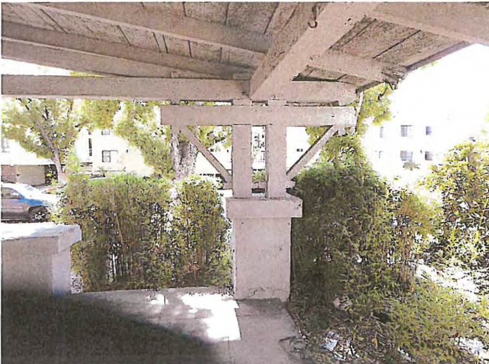
Photograph 3: Detail of double kneebraces, pegged joinery, massive purlin (center top) and open truss (left side) at front porch. May 2019.
