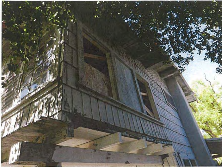
Figure 3. Detail of Rear Second Floor Addition, 534 N. Kenwood SOURCE: Sapphos Environmental, Inc., 2017
