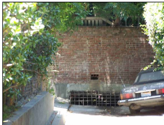
Figure 18 (left) View looking west at the inlet (covered by a steel grate) to an underground Los Angeles Flood Control District drain pipe
