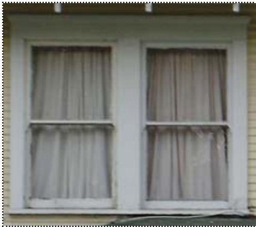
Above: Paired wood double-hung sash with notched corners. The simple flat wooden surrounds are typical.
