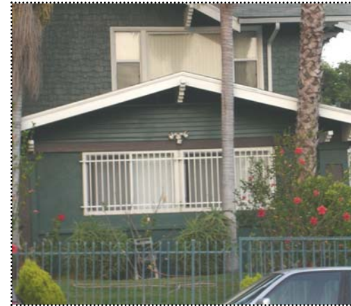
Above: The enclosed porch on this house detracts from the structure's historic value.
