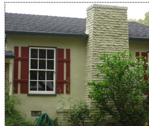
Below: This stucco house has a brick chimney with untooled mortar joints, an effect known as "weeping" mortar.
