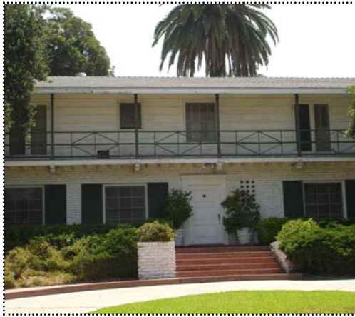
Above: The eave for this roof provides little overhang. The roof cladding is composition shingle.
