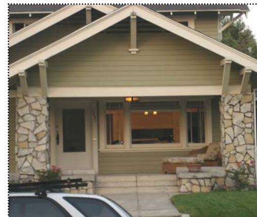
Below: The flagstone supports of this porch are inappropriate to the Craftsman style and should be replaced with its original materials.
