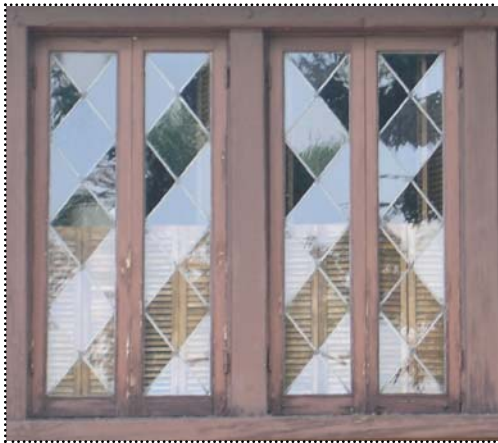
Above: These leaded casement windows are a very important component of the front facade of this house.
