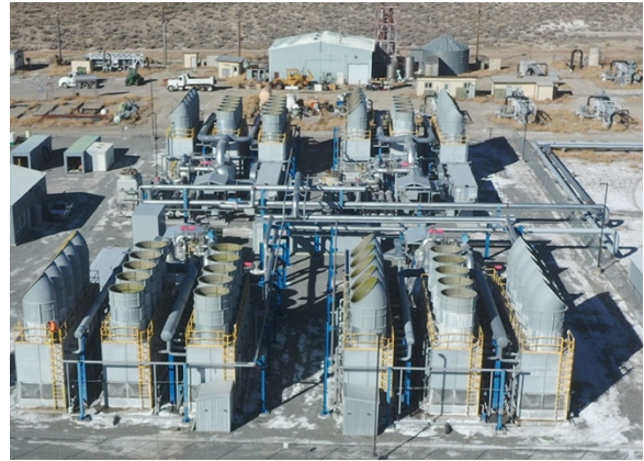
Figure 20. Whitegrass No.1 Geothermal Plant
