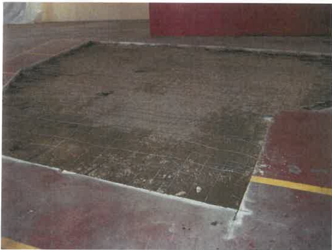
Photograph 4: View of backfilled excavation pits in Bays 1 and 2 prior to concrete replacement.
