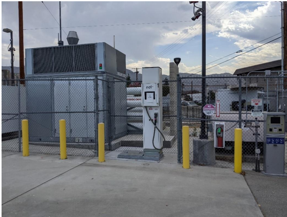
Figure 1-10: Light-Duty Hydrogen Fueling Station at 124 South Lake Street, Burbank, CA (Source: CALSTART)
