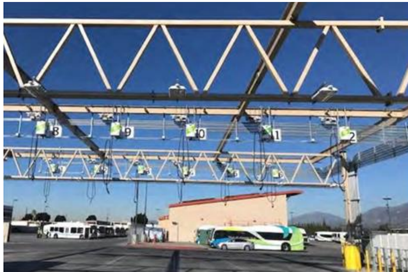
Figure 1-5: Overhead Plug-in Charging Example (Source: Burns McDonnell Foothill Transit In-Depot Charging and Planning Study)
