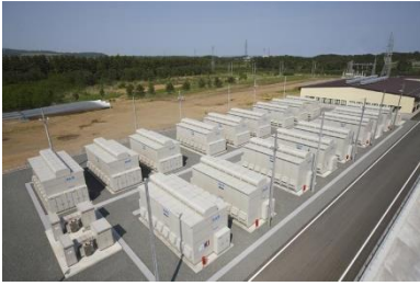
NGK NAS Battery System
