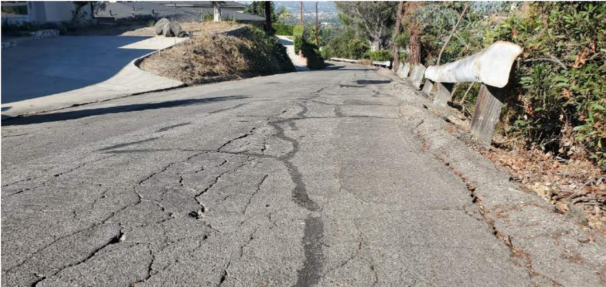
Figure C-10 – AC pavement cracks, cracked and settled berm, and leaning guardrail posts in front of 340 View Crest Road (provided by the City)
