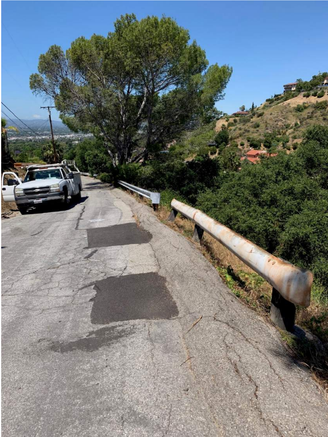
Figure C-17 – Cracked and settled berm and leaning guardrail posts in front of 346 View Crest Road.
