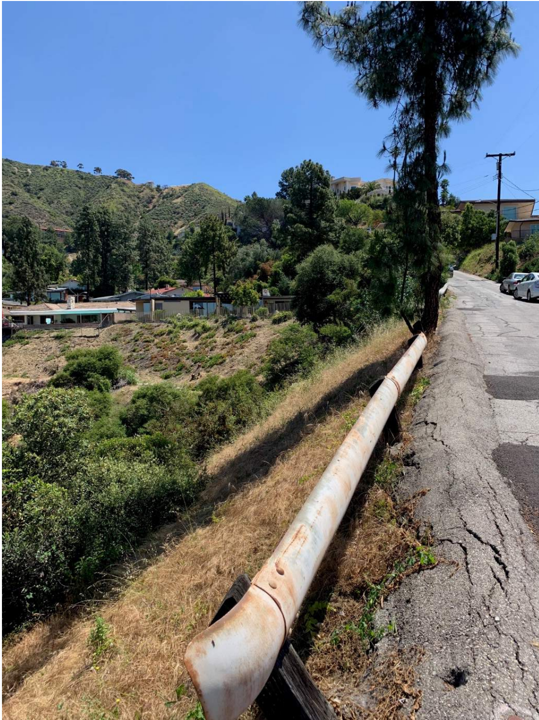
Figure C-16 – Cracked and settled berm and leaning guardrail posts in front of 346 View Crest Road.
