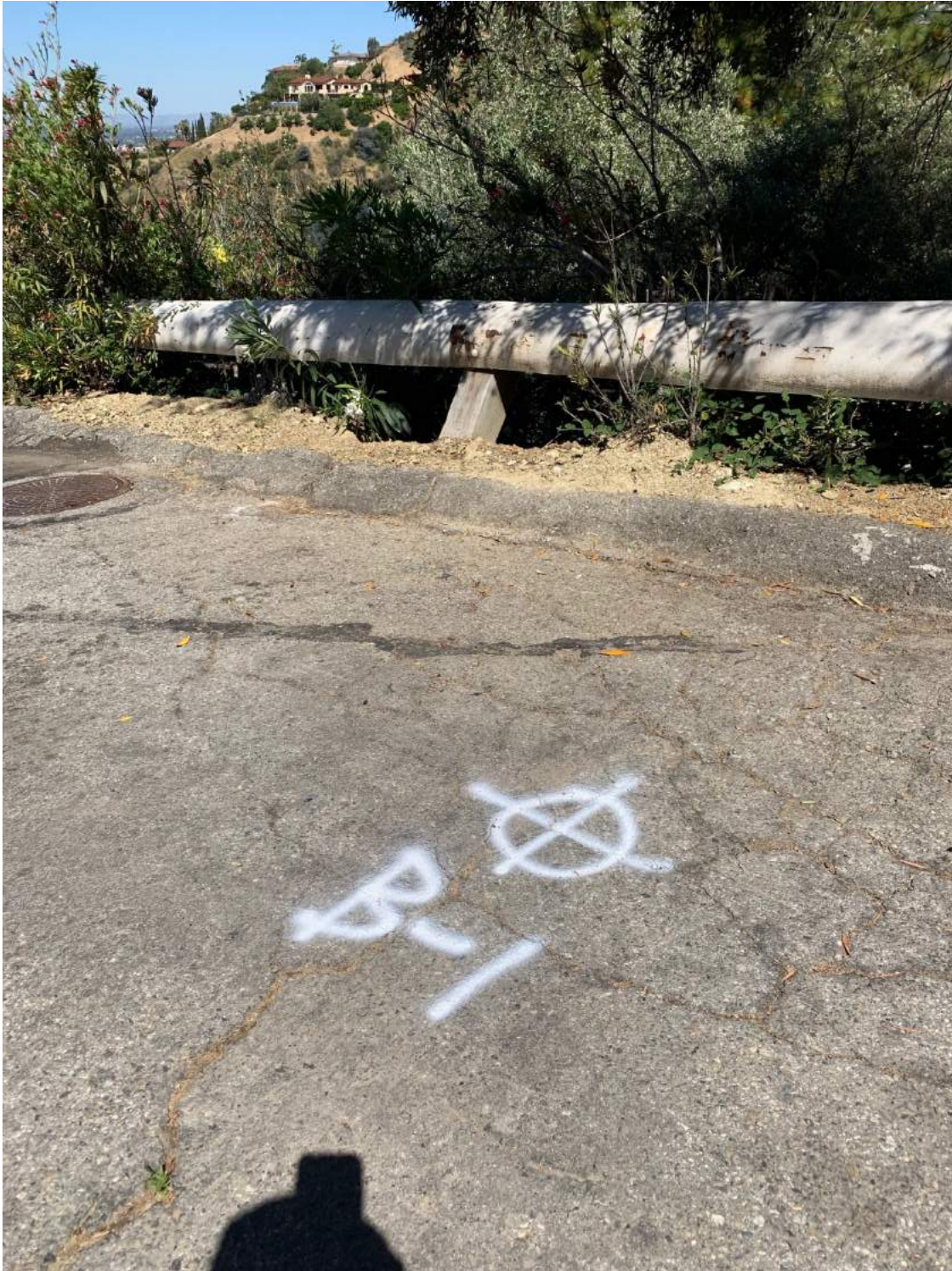
Figure C-4 – Pavement alligator cracks, leaning guardrail posts, and vegetation in front of 306 View Crest Road
