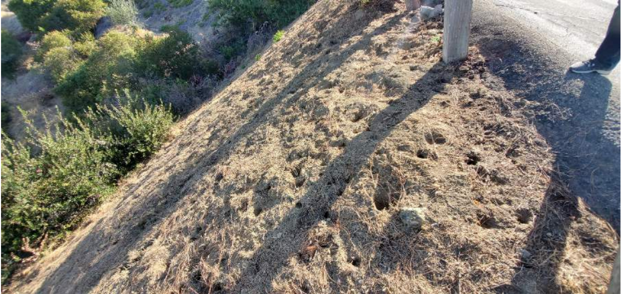
Figure C-12 - Rodent holes in slope in front of 340 View Crest Road (provided by the City).
