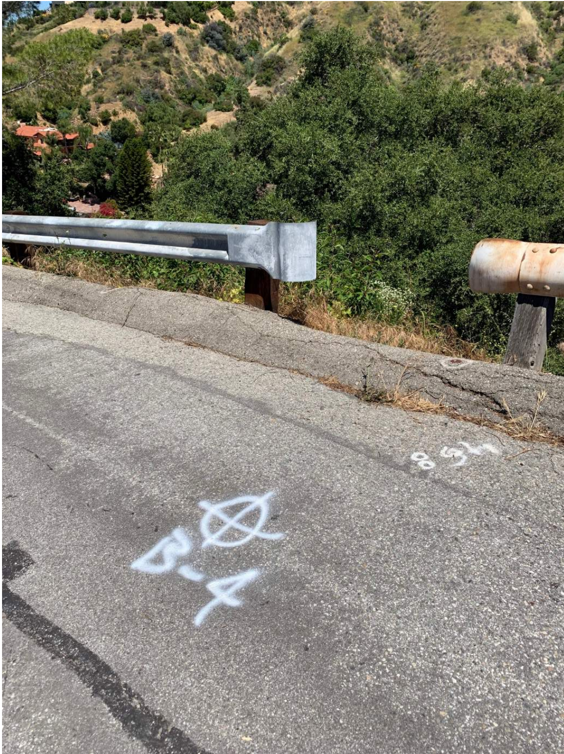
Figure C-15 – Cracked and settled berm and leaning guardrail posts in front of 346 View Crest Road.
