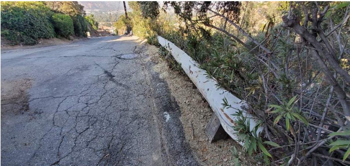
Figure C-3 - Cracks around sewer manhole in AC pavement and berm and leaning guardrail posts in front of 306 View Crest Road (provided by the City)
