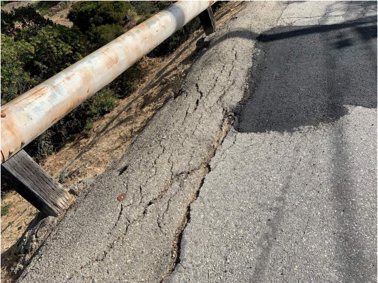
Figure C-18 – Leaning guardrail posts, cracked and settled AC berm and pavement in front 346 View Crest Road.
