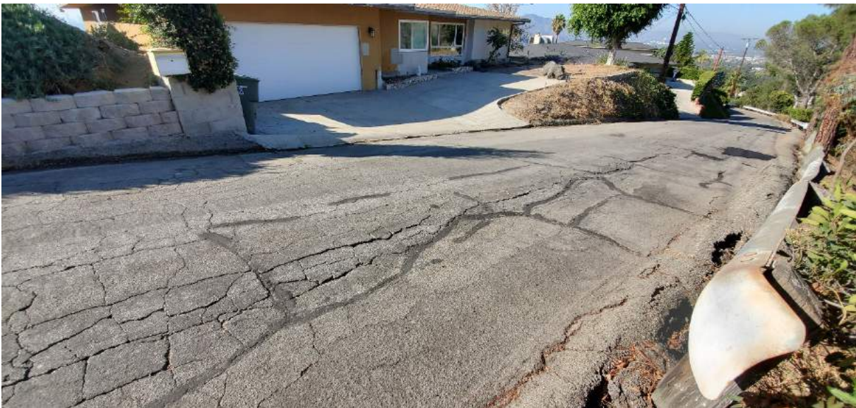
Figure C-11 - Cracked AC pavement, failed berm, and leaning guardrail posts in front of 340 View Crest Road (provided by the City).
