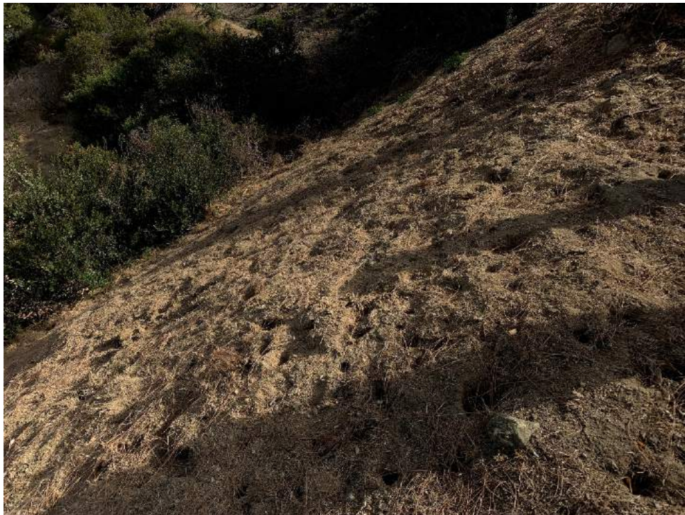
Figure C-13 – Rodent holes in the slope in front 340 and 346 View Crest Road
