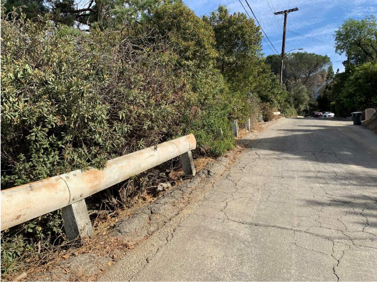
Figure C-6 – Cracked and settled berm and pavement cracks in front of 326 View Crest Road
