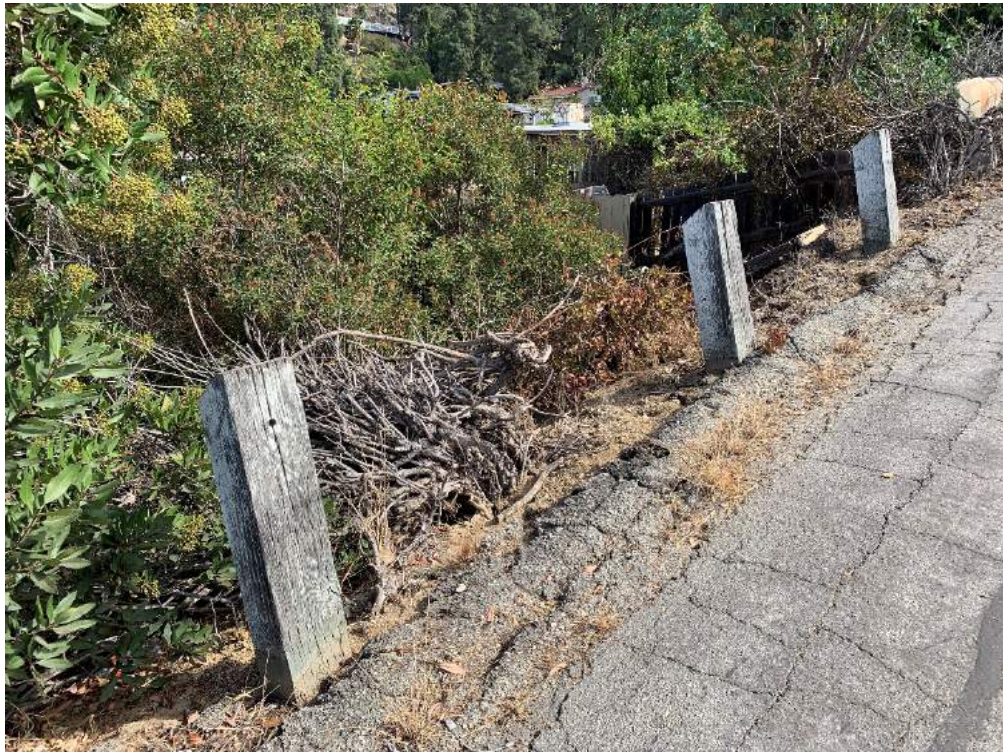
Figure C-9 – AC berm failure and pavement alligator cracks in front of 330 View Crest Road.
