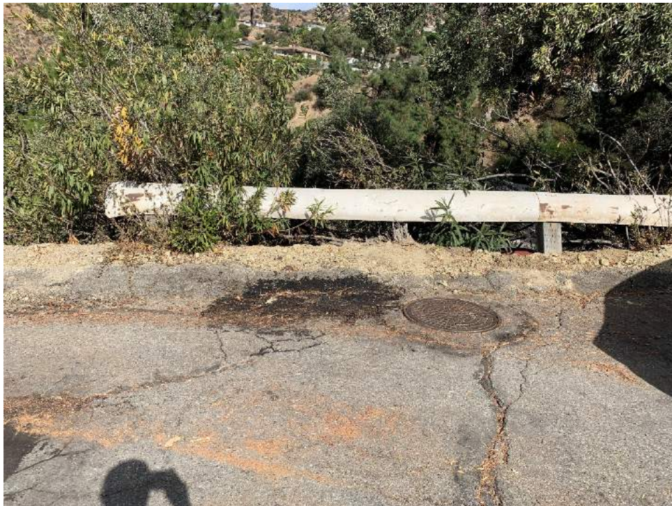
Figure C-5 – Pavement cracks and leaning guardrail posts around the sewer manhole in front of 306 View Crest Road
