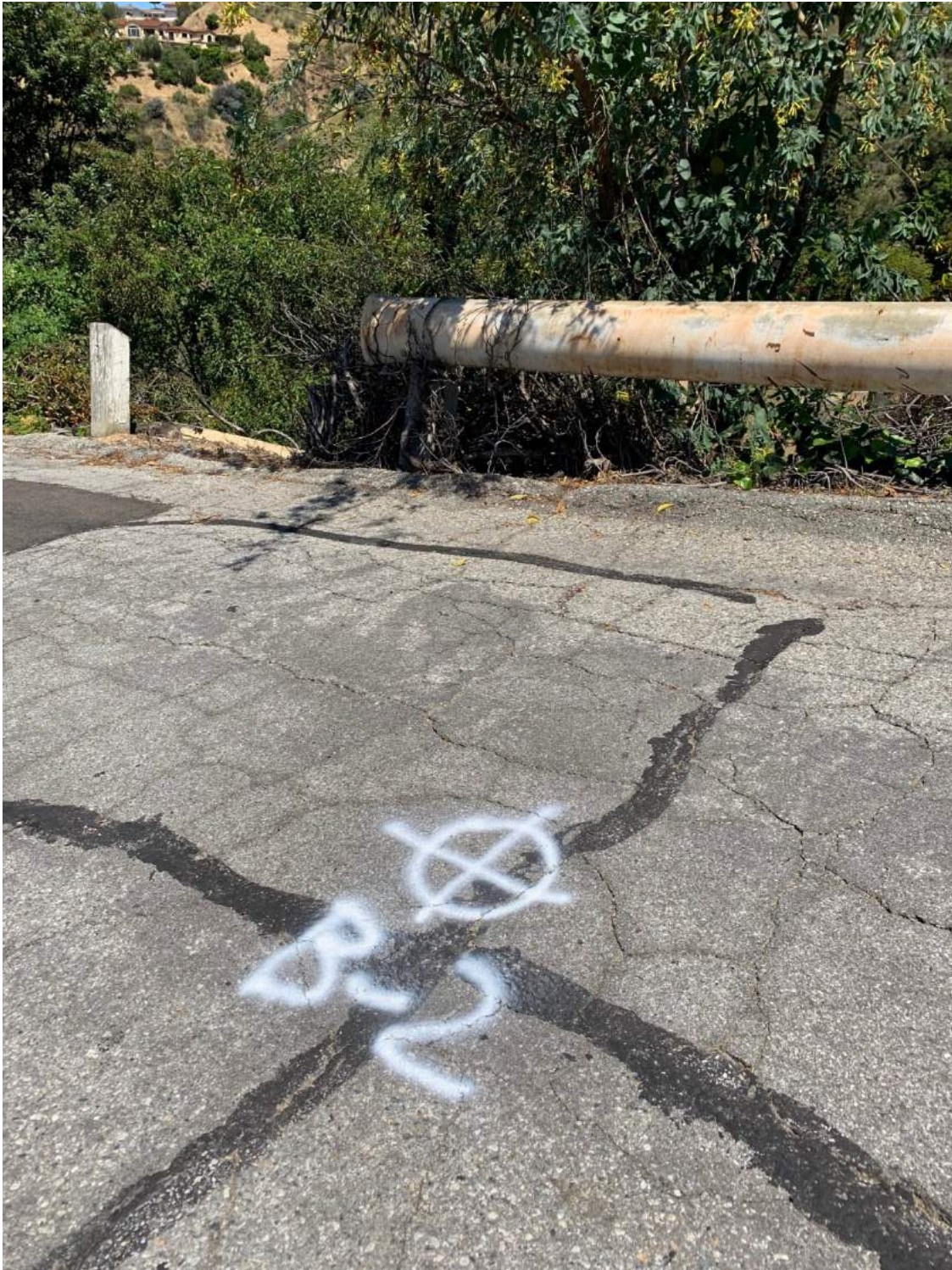
Figure C-7 - Pavement alligator cracks, cracked and settled berm, and vegetation in front of 330 View Crest Road
