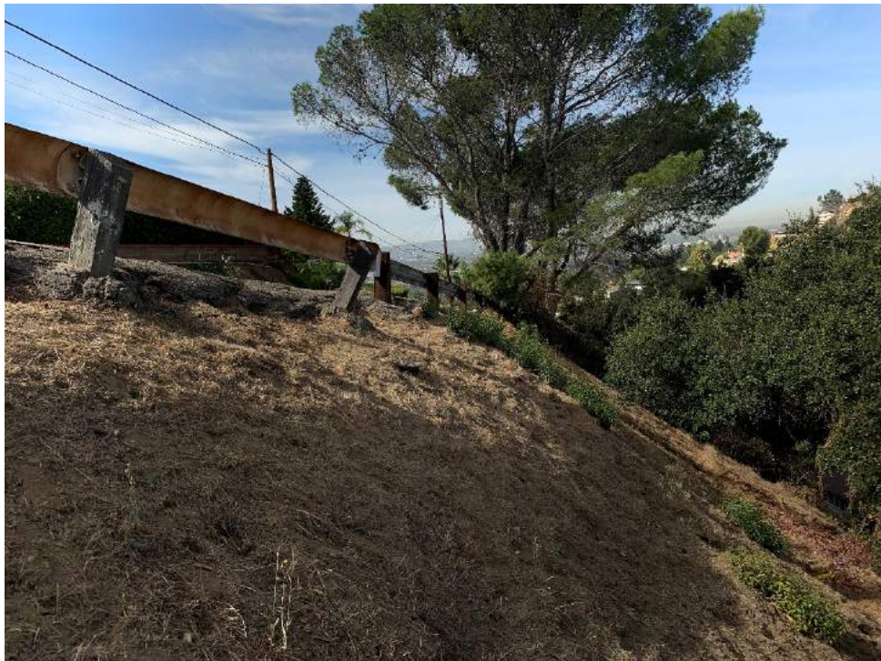
Figure C-14 – Rodent holes in the slope in front 340 and 346 View Crest Road
