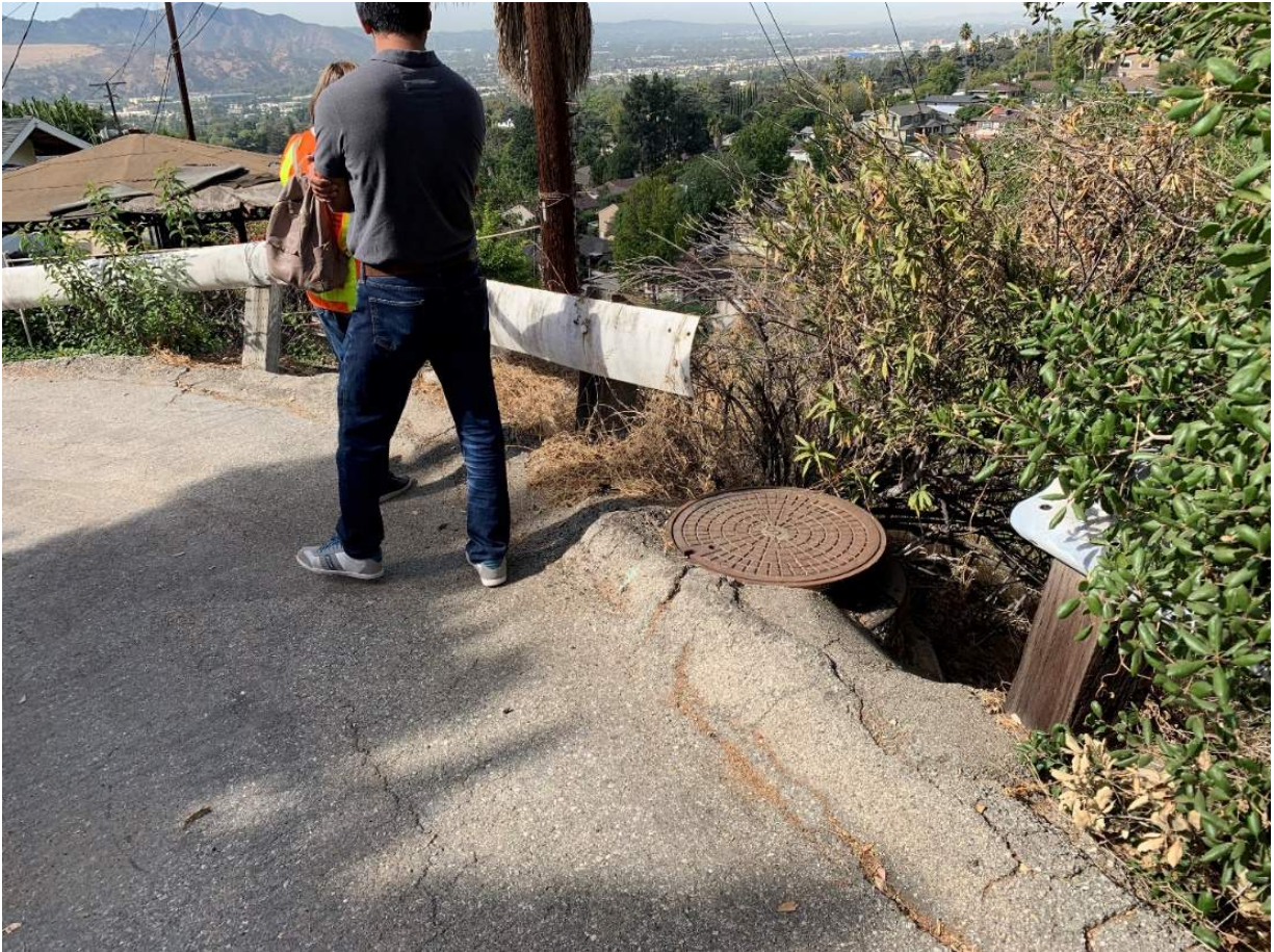
Figure C-19 – Berm failure around sewer manhole in front 354 View Crest Road.
