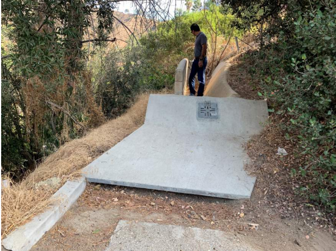
Figure C-2 – Stormwater ditch at east end of View Crest Road near 306 View Crest Road
