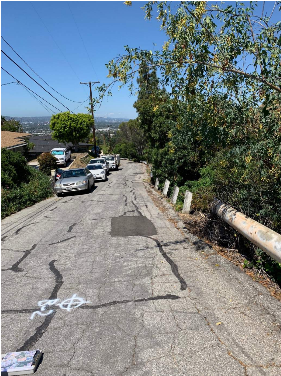
Figure C-8 – Pavement alligator cracks, berm cracks and settlement, and leaning guardrail posts in front of 330 View Crest Road
