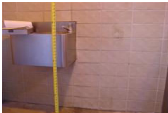
Men's Restroom Next to the Play Equipment Citations: ADAAG 4.19.2
