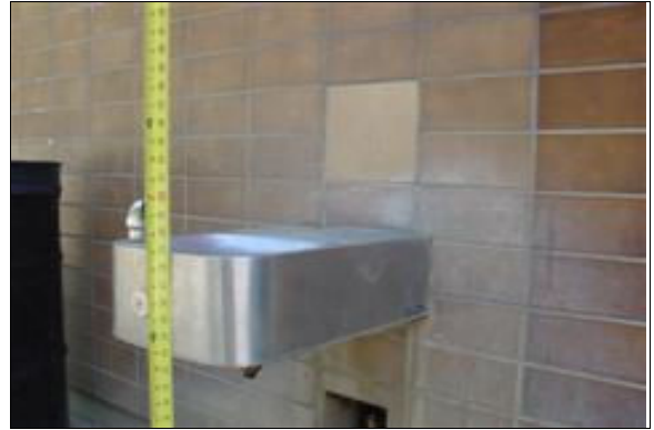
Drinking Fountain at the Restrooms Next to the Play Equipment
