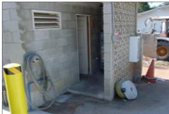
Unisex Restroom at the Maintenance Yard
