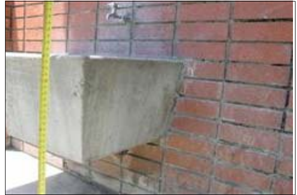
Sink at the Outdoor Dining Area
