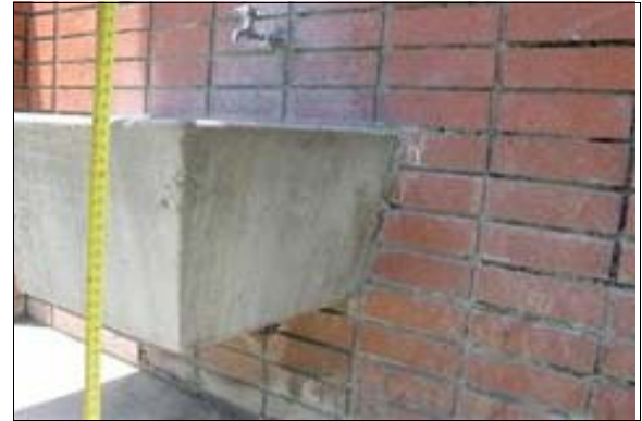
Sink at the Outdoor Dining Area
