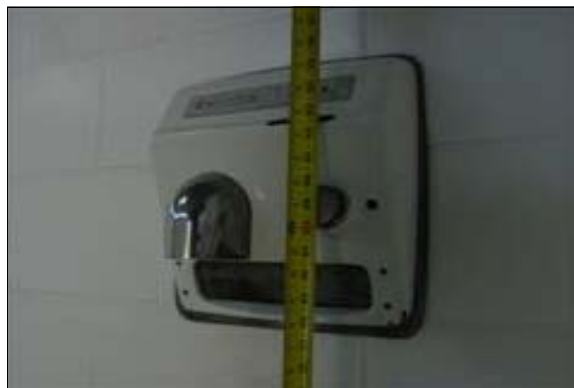
Men's Restroom Next to the Play Equipment Citations: CBC 1115B.9.2; ADAAG A4.27
