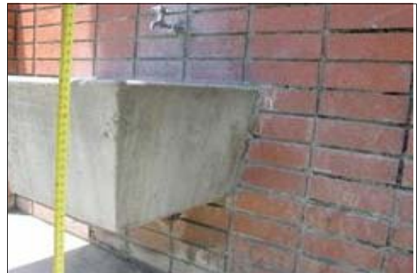
Sink at the Outdoor Dining Area
