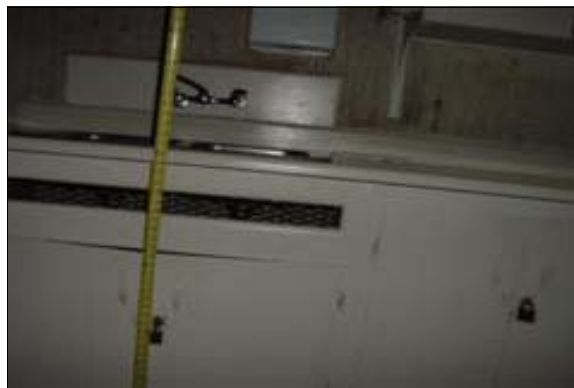
Sink in the Community Center
