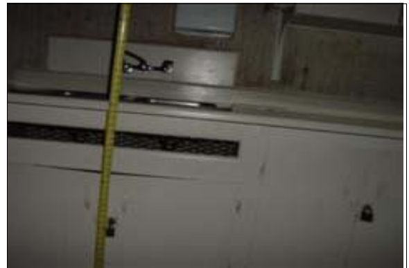
Sink in the Community Center
