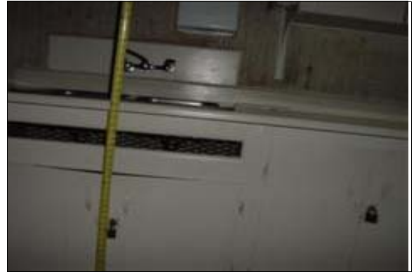
Sink in the Community Center
