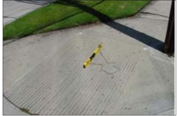
Curb Ramp off of Verdugo (Center Left)
