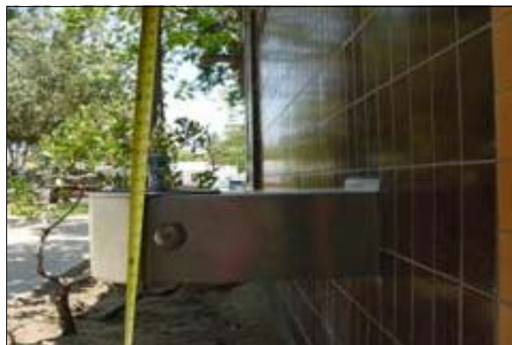
Drinking Fountain at the Restrooms
